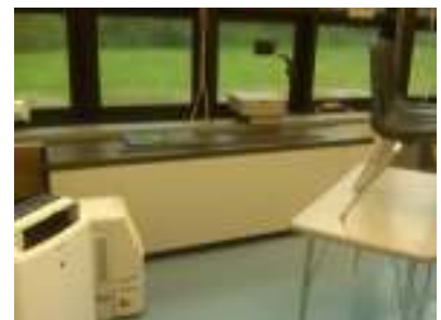
Figure 1 Classroom 120. Pictured is unit ventilator where AtmosAir unit is integrated into.
